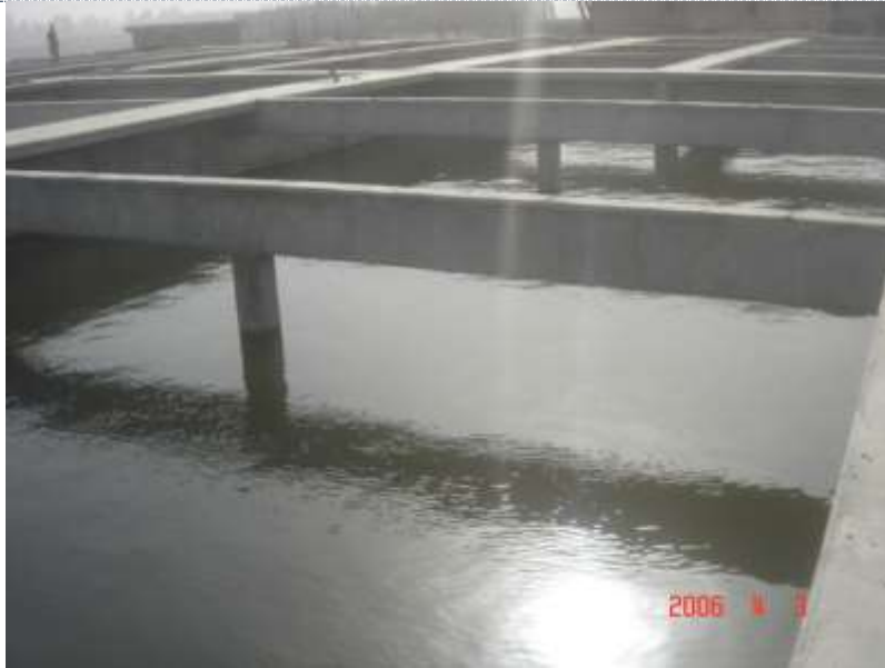
Figure 2: Photo of Alkurech sedimentation tank.
